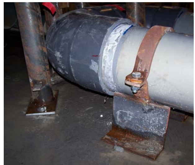
b) Damaged PVC U-bend at distance x = 125.5 m.
