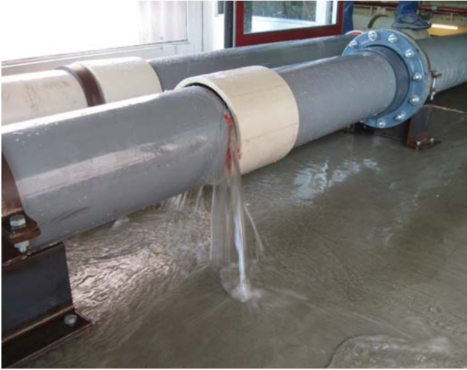
a) Leakage from damaged PVC pipe joint at distance x = 257.2 m.
