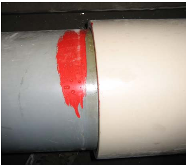
a) Damaged PVC pipe joint at distance x = 119.1 m.
