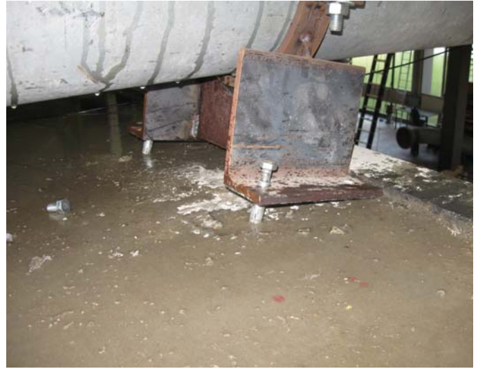
b) Damaged metal anchor at distance x = 260.6 m.
