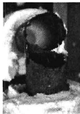
figure 3.39: broken radiant tube
