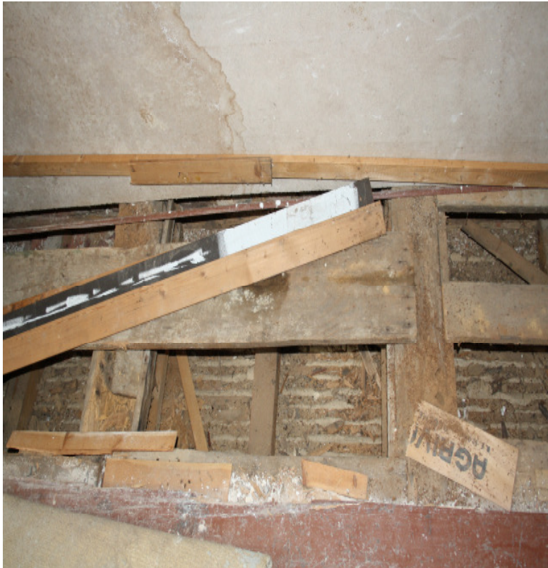
Figure 3.20: Destroyed beam ends in an area of the roof over the ground floor
