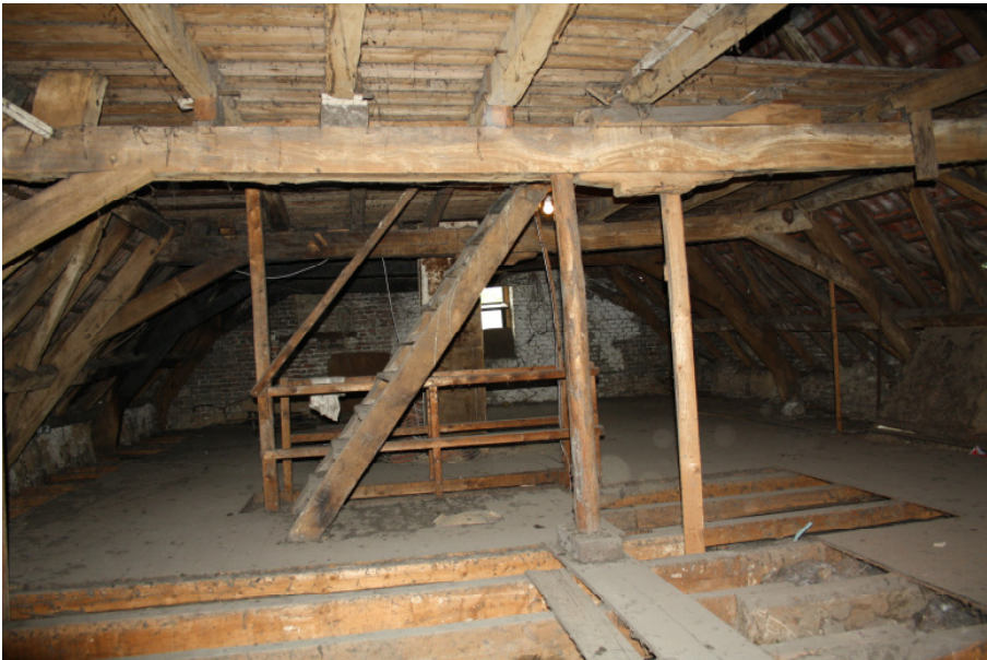
Figure 3.14: Photo – Level 1 of the roof construction (line of sight from front to back)
