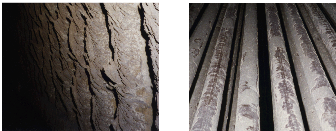
Figure 2.3 Deposits observed on the tubes in the final superheater C (left picture) and in the economiser F (right picture) of the boiler in Moerdijk.
