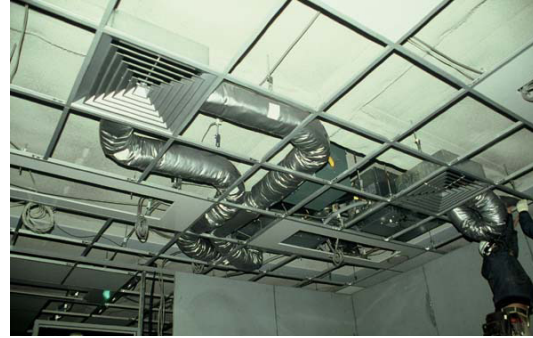
Figure 6. Ceiling and mechanical equipment
