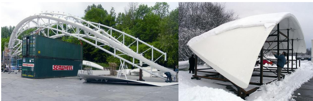
Figure 6. Test assembly of the central body and lower wing of the Library in Lelystad
