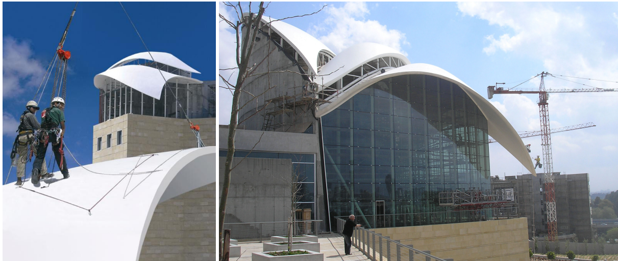
Figure 7-8. Montage of the GRP sandwich roofs in October 2005 (left) and the Great Hall in April 2006
