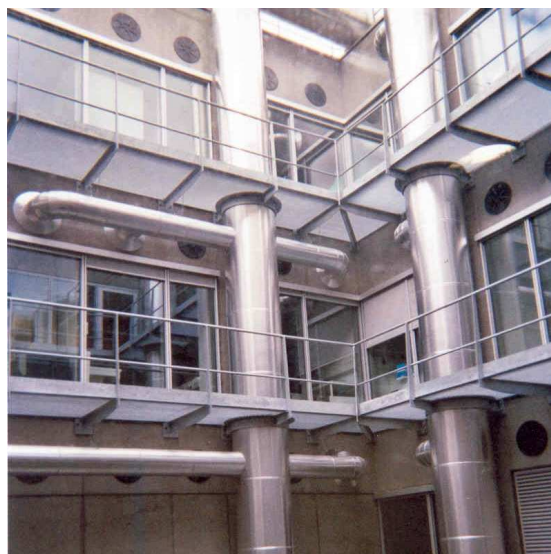
Fig. 2 Flexibility of the structure: Service ducts can be adapted and can cross the concrete beams
