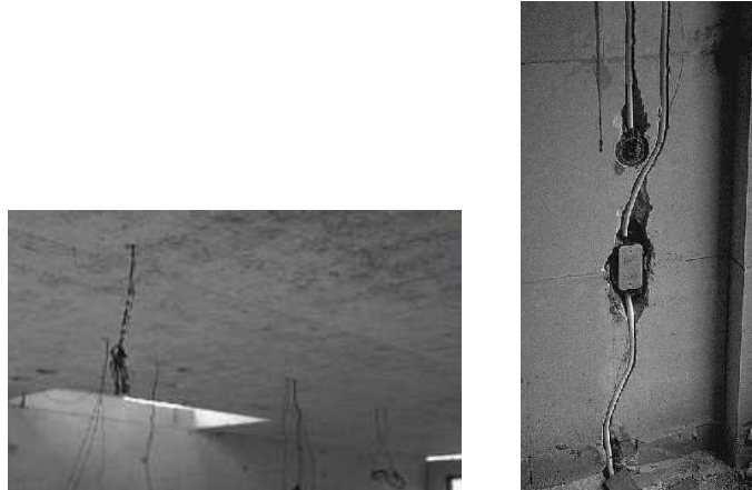
Figure 1. Cables and pipes housed in weight-bearing floors (left) and walls (right): not adaptable
