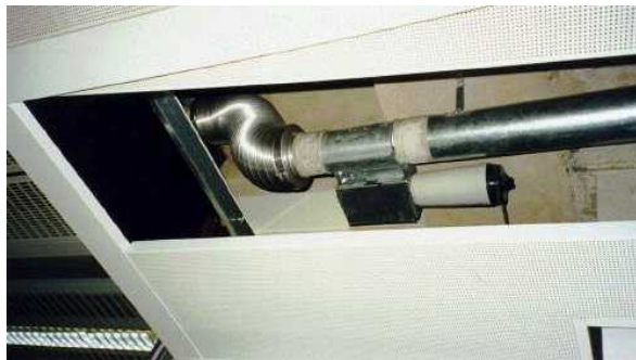
Figure 4. Distribution ducts and control facilities in an easy-to-dismantle ceiling
