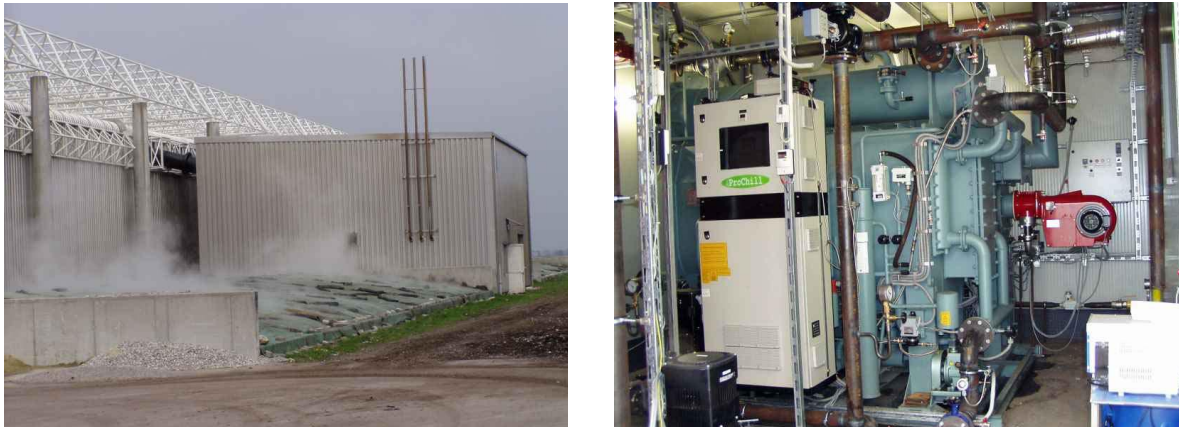
Figure 1 left: Composting hall, which is used as heat source, the machine hall where the low temperature heat is exchanged from the air to the water of the evaporator circuit and the bio filter in the front of the photo, right: the absorption heat pump
