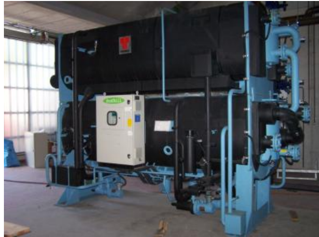
Figure 4: Picture of the absorption heat pump at Ackermannbogen
