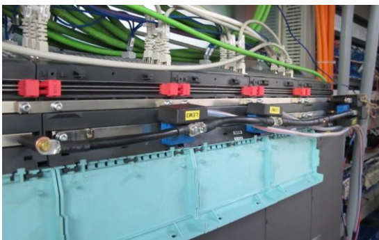
Figure 3: Mounted Hall-effect current sensors for measurement on the DC link to drive inverters.
