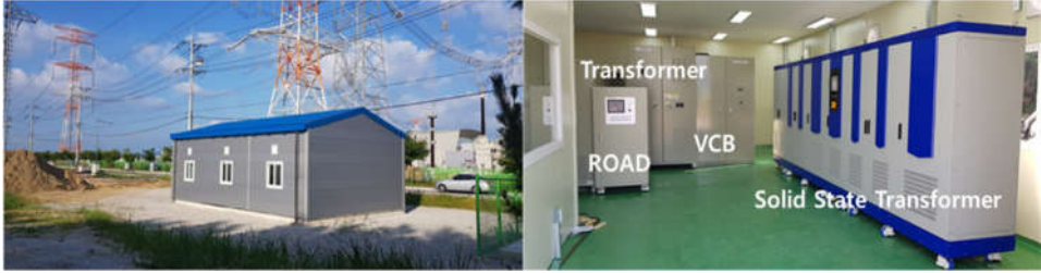
Figure 11-26 Conventional transformer used for powering MV electronics [36]
