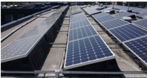
(a) South-facing panels
