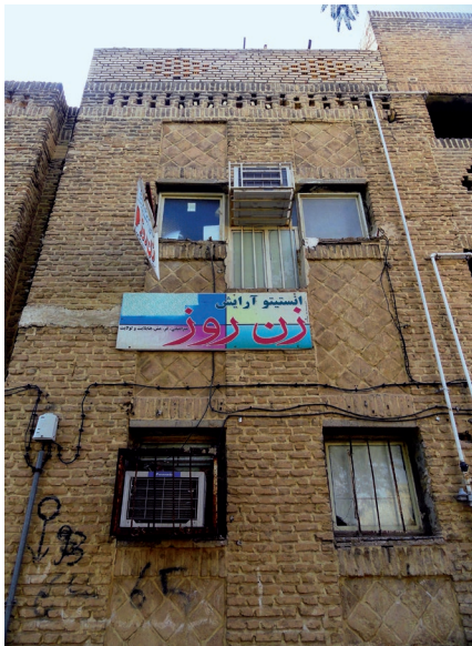
Fig. 34: Gas pipes, ventilators, and advertisement signs have been installed carelessly (Author)
