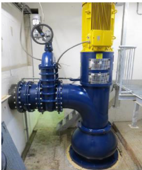
Fig. 12 Fish friendly vaned diffuser in Obdam pumping station in The Netherlands
