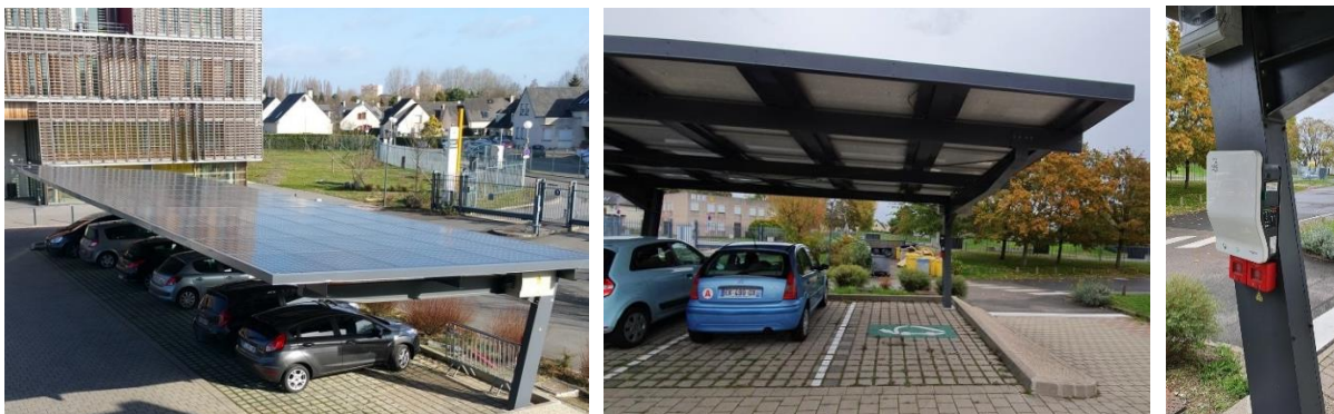
Fig. 4.3-12 PV-powered charging infrastructure with PV vehicle parking shade
