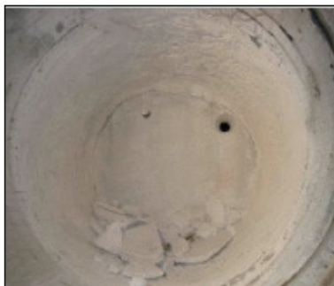
Figure 1.7: An example of a monolithic steel ladle bottom in which the refractory lining has exploded (steam spalling) due to an improper heat-up procedure.
