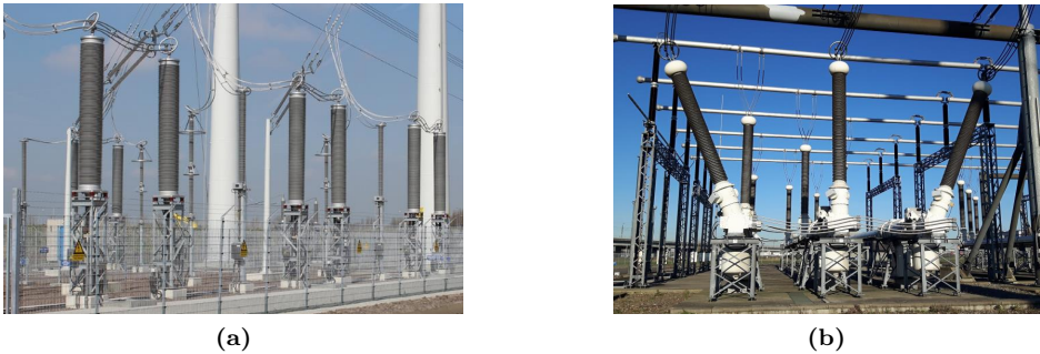
Figure 5.7: (a) Representation of the transition point configuration; (b) configuration of one circuit at substation BWK.
