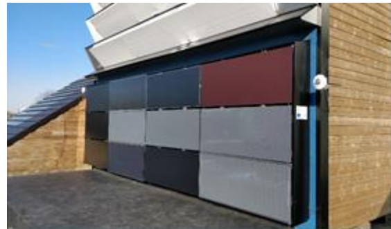
Figure 2: The outdoor colored and textured PV façade demonstrator installed at SolarBEAT, Eindhoven.
