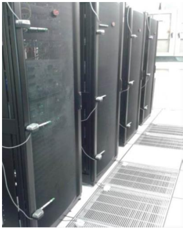
Figure 3 Illustrative picture of the demo DC site in Cork (Ireland)
