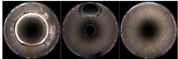
Figure 1. Forward-facing pictures of the same concrete sewer pipe at different locations along the street.
