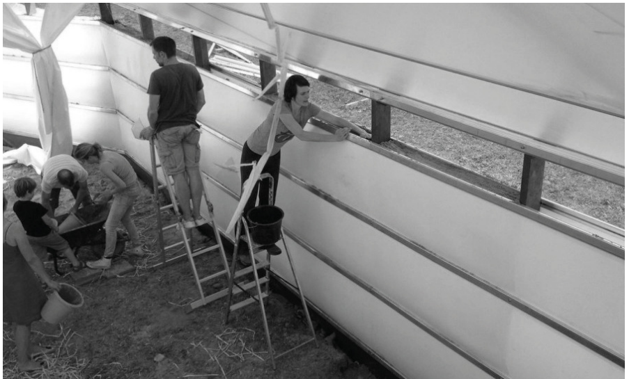
P19. A team of people building the Maggie Shelter. The inner core is being filled with a mixture of sand and straw
