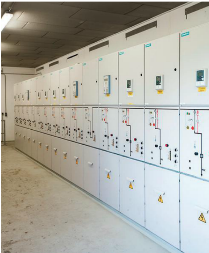
A medium-voltage switchgear installation equipped with distribution automation and protection relays, showing different relay and switchgear indications.
