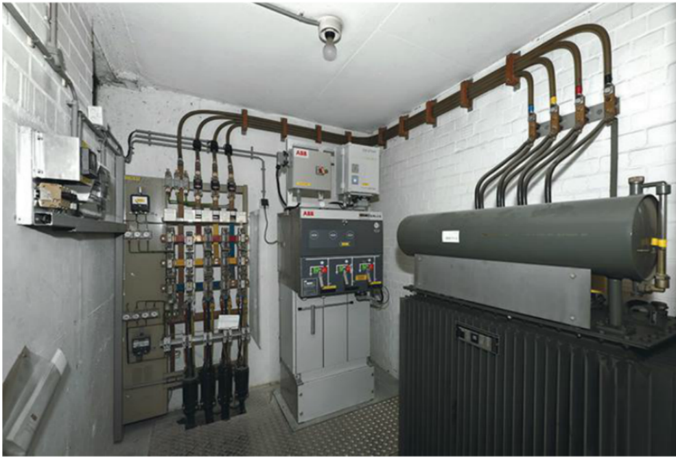
This is a typical Enexis medium-voltage/low-voltage indoor substation that includes a MV/LV distribution transformer, MV switchgear and a LV distribution board that has been upgraded to include distribution automation.
