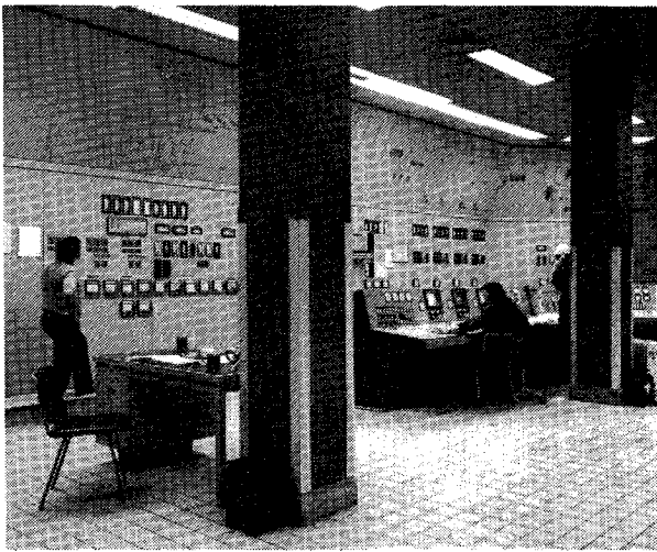
Fig. 3. Control room of fertilizer plant.
