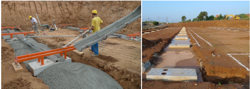
Figure 16. Steel supports help to position slabs accurately. Figure 17. Beams and tie beams that have already been concreted.
