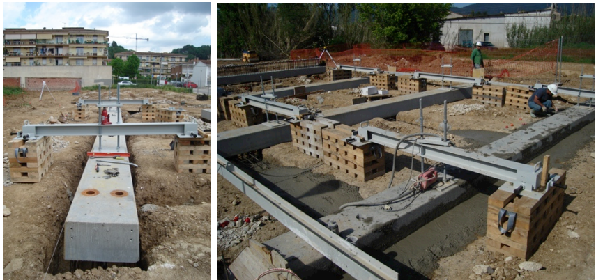
Figure 12. Suspension of partial prefabricated beams to be completed with in situ concrete. Figure 13. Concreting of the lower part of the partial beams and of the tie beams.
