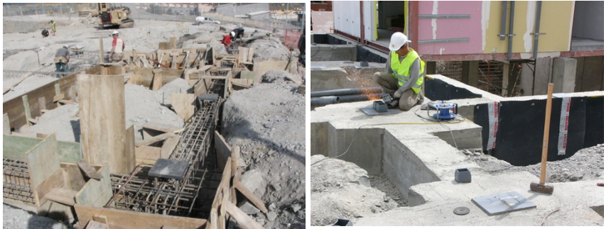
Figure 10. Reinforced and shuttered footings, tie beams and plates for connection to the modules. Figure 11. The cutting of offset connector bolts with a grinder.
