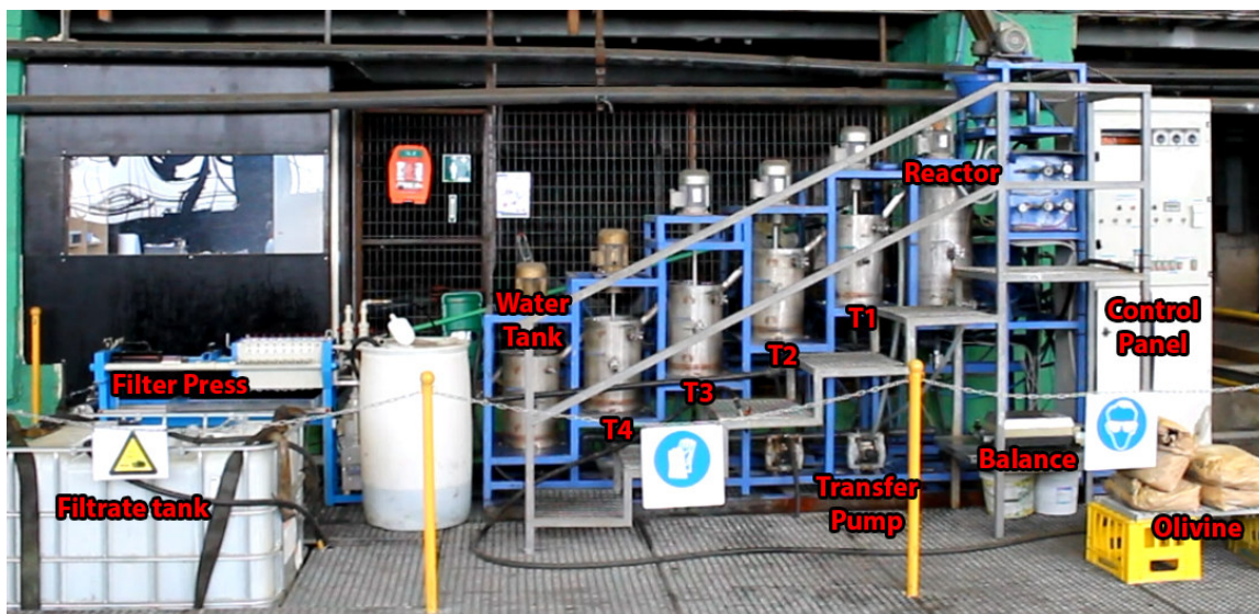
Figure 9.11. Picture of the production pilot plant in Hellas Gold (Greece) [173].
