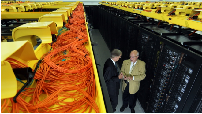
Figure 1.2: View from the top of IBM’s SuperMUC supercomputer installed at Leibniz Rechenzentrum (LRZ) in Munich, Germany in 2012. Image is a courtesy of IBM Research - Zurich. The orange wiring on the top are active optical cables linking compute nodes and storage servers [3].
