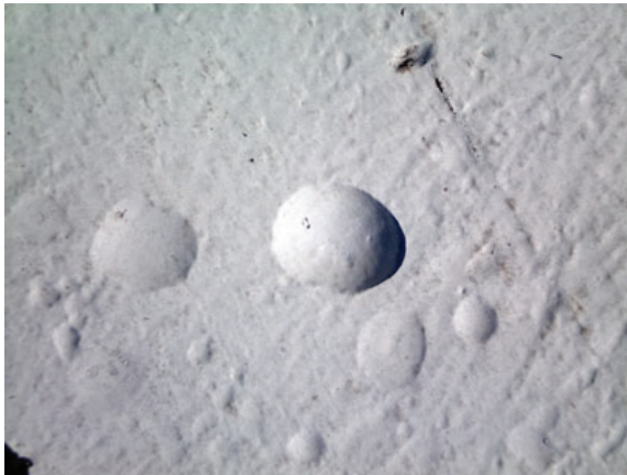
Fig. 1.5: Blisters under coatings as a typical damage by water.
