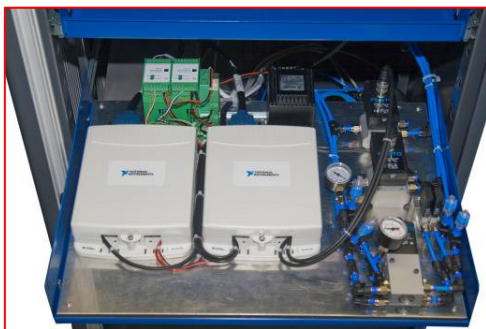
Fig A.3: The electronic and pneumatic components are mounted on a plate attached to a sliding drawer
