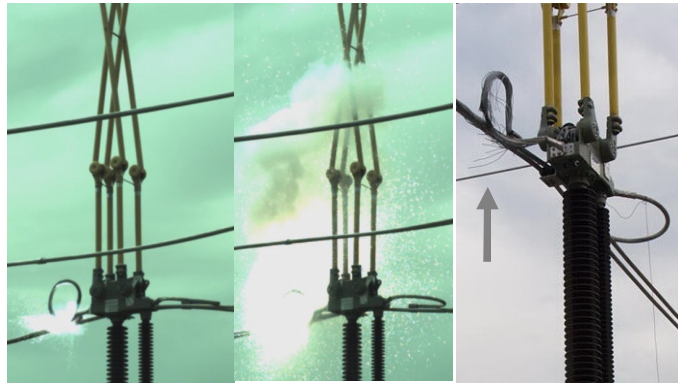
Fig. 17: Severe arcing at 80 kA test on flexible disconnector connection loop and resultant conductor damage (right).
