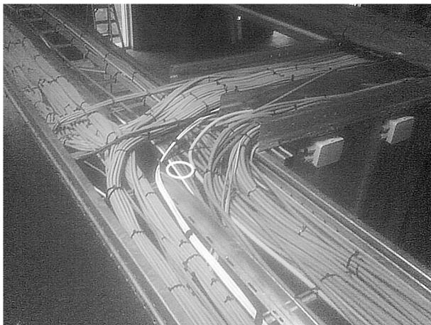
Fig. 3. Photograph of connection of three cable ladders. The white ellipse emphasizes the four test cables.
