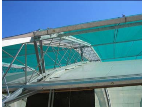
Fig 2. Detail of the roof, the truss structure and the upper and lower foil
