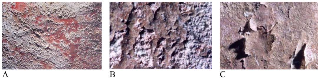
Figure 4 A-C: Hardham Church, West Sussex, England: Detail of wall paintings: showing damage due to salt crystallisation and organic coatings (photo: A. Heritage, Conservation of Wall Painting Department, Courtauld Institute, 1994)
