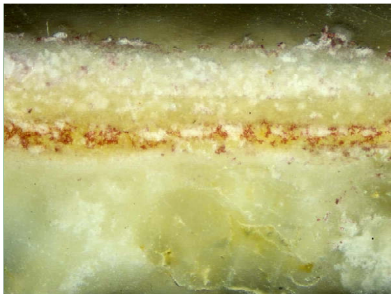
Figure 5. Hardham Church, West Sussex, England: Photomicrograph (200x magnification) of cross section taken from nave south side, after histochemical test for sulphate. Gypsum (identified by areas stained purple) is present solely within a yellow layer of wax (dated to 1934) between the original plaster and a surface limewash dated to 1935. (photo: A. Heritage, Conservation of Wall Painting Department, Courtauld Institute, 1994)
