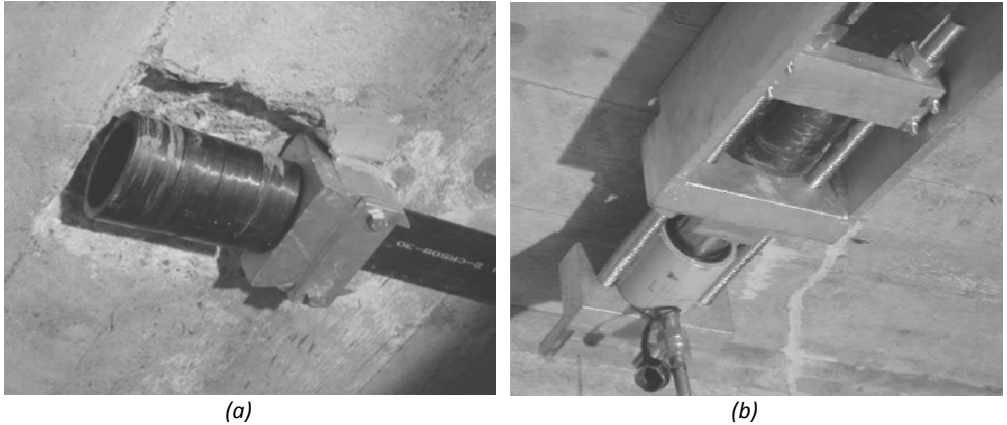
Figure 2-10: Fixed (a) and movable (b) end anchor with hydraulic jack to apply the prestress to the FRP (SIKA Stress-Head system)
