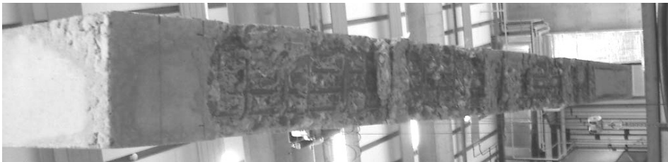
Figure 7-22: Internal steel reinforcement is clearly visible after concrete cover rip-off
