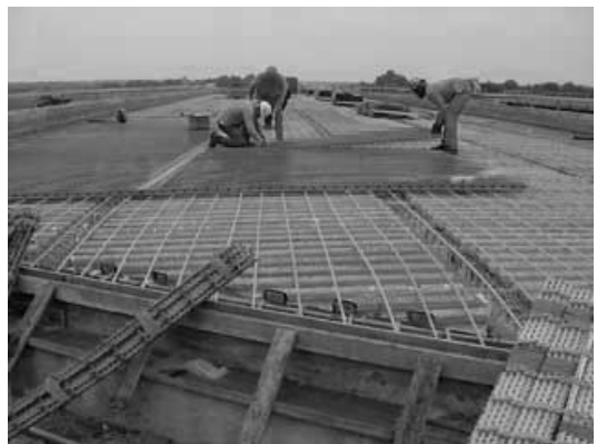
Figure 2-4: Application of GFRP reinforcement bars in a bridge deck in Canada (Hughes Brothers 2007)
