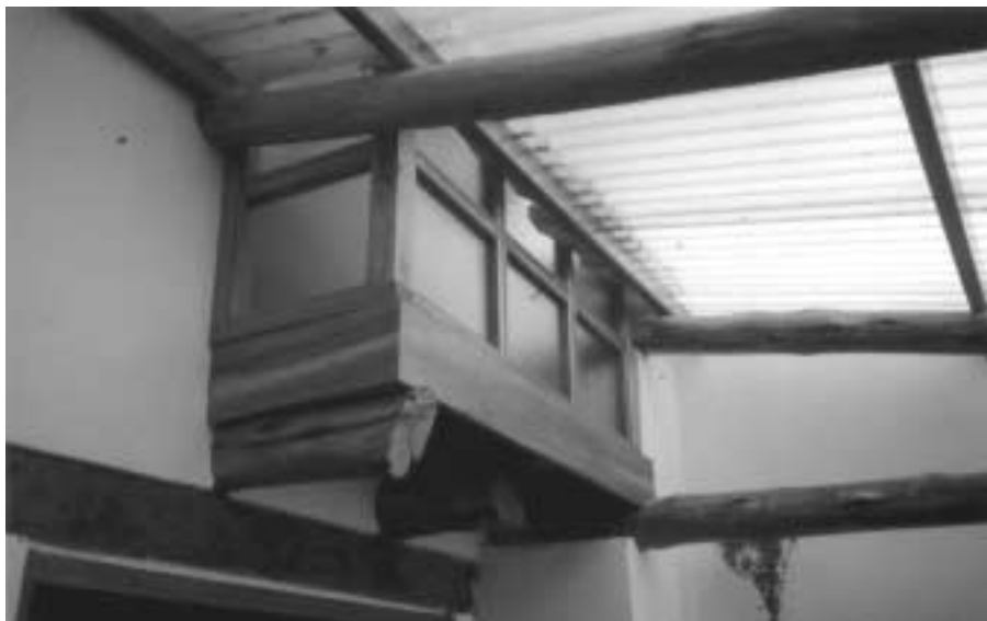
Fig. 1. Errors in the construction due to bad planning (Photo Erkelens)
