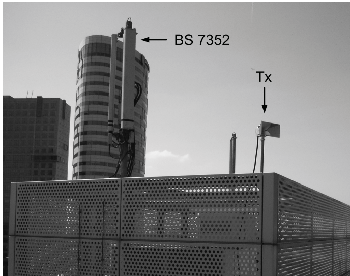
Fig. 5.4: Transmitting antenna positioned outside, close to BS 7352 and pointed in the same direction.
