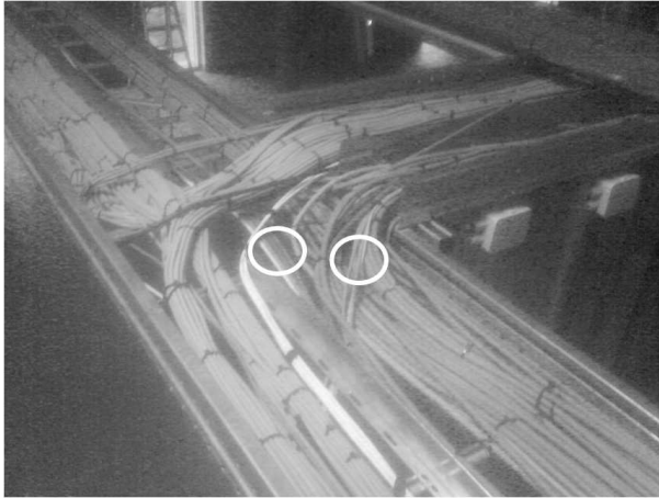
Figure 2.3: Photograph of connection of three cable ladders. The white ellipses emphasizes the two test cable bundles.
