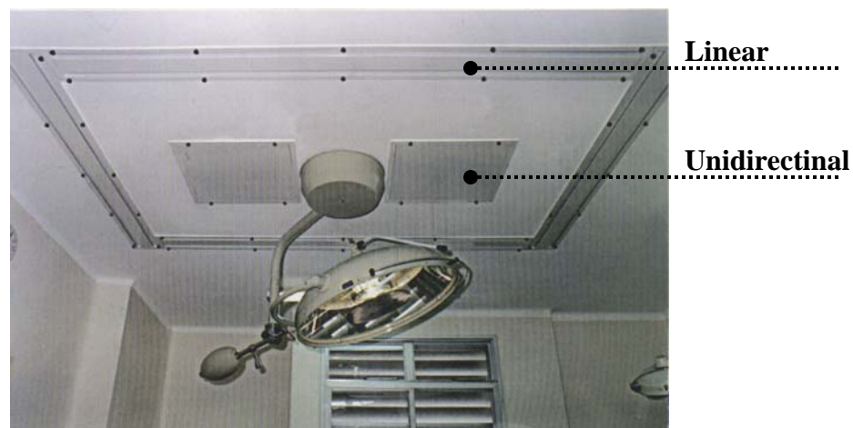
Figure 6. Example of Unidirectional and linear systems (TROX do Brazil, 1992 - reported by Melhado, M. 2003)
