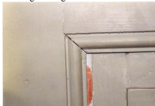
Figure 4. One of the panels hanging loose in the frame
