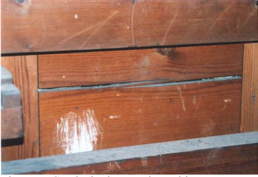
Figure 5. Cracks in the wooden cabinet
