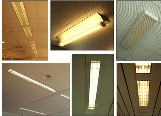
Figure 3.9 Different types of electric lighting
