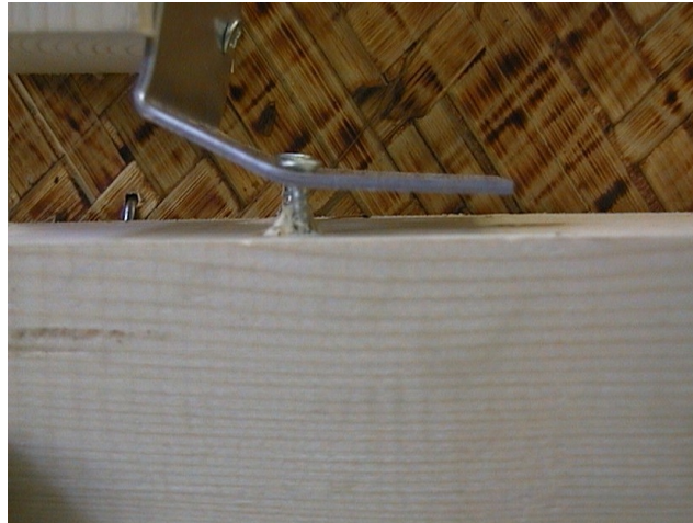
Figure 5-10 Ultimate failure in connection between the vertical member and the lower soleplate using mat boards.
