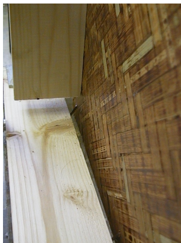
Figure 5-9 Failure in test MB1 due to the high deformation of the nail in the corner. The vertical member is not joined to the lower soleplate.
