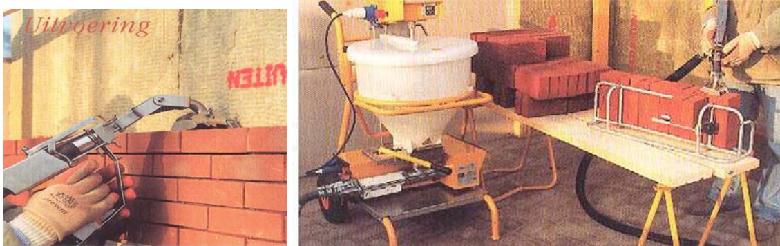
Figure 9 Execution of thin layer masonry using a stand to mortar the unit headers.
