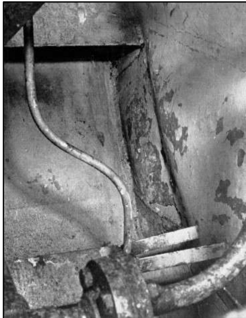
Figure 3.12 Buckling of a bulkhead caused by a non-contact UNDEX explosion (Keil [3.7])
