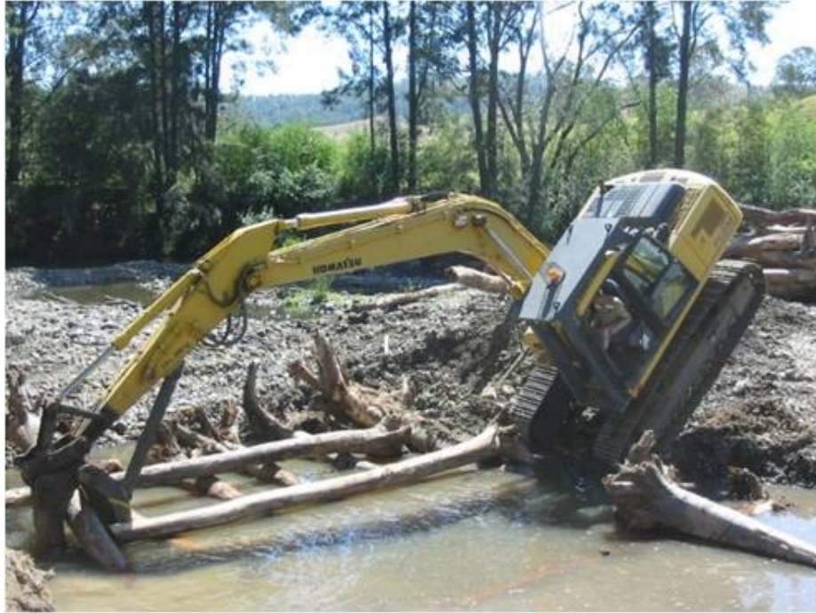
Plate 2.1 Constructing the ELJ that anchored the upstream log sill into the right bank at WUM. Note that the channel was dammed upstream of the riffle and the river bed excavated to place the logs.
