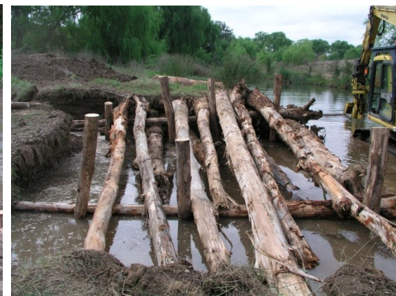
Plate 2.6 The 'bank deflector jam' on the right bank upstream of the first log sill. Its purpose is to deflect flow from the head of the gravel bar on the right bank to prevent the upstream log sill from being outflanked during high flows.
