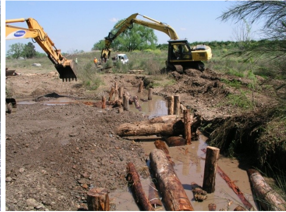
Plate 2.4 The upstream log sill at HGB. Note the right channel has been dammed to the right (upstream) of the ELS. The ELS consists of the cross-spanning logs, the supporting abutment jams and the piles. Photo was taken from the central island looking towards the right bank.
