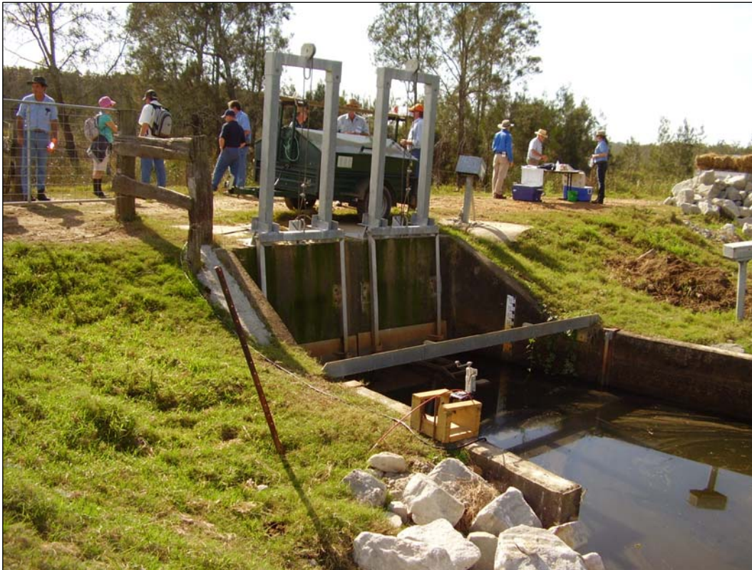
Photo: Floodgate for regulating tidal exchange at the Little Broadwater Wetland on the Clarence River floodplain, May 2007.
