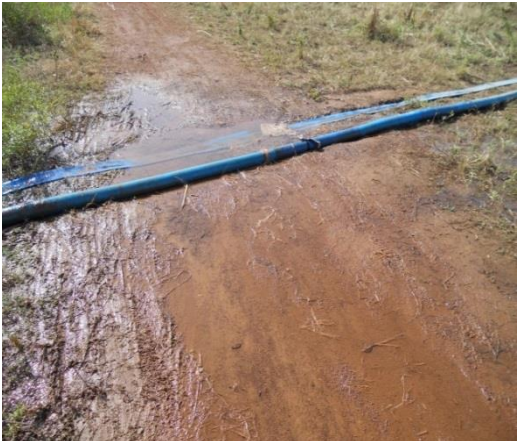
Water leaking from broken pipes, Durongo
