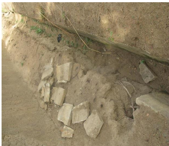
Collapsing canal wall, Winkogo
