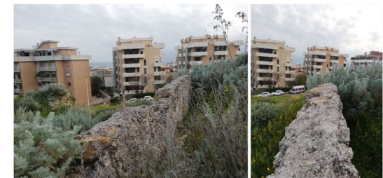
Fig. 10 - Wide views captured with drone flight and detail captured from the ground of the portion of a vertical connecting structure (R1 in figures 19-22) positioned between the fort of "Sant'Ignazio" and some additional works designed to control the route located between the hill of "Monte Urpino" and the hill of "Montisedu".
