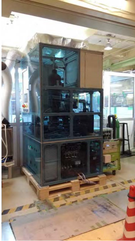
Figure 90. MARCO cooling system installed in the Tsukuba hall B4 floor.
