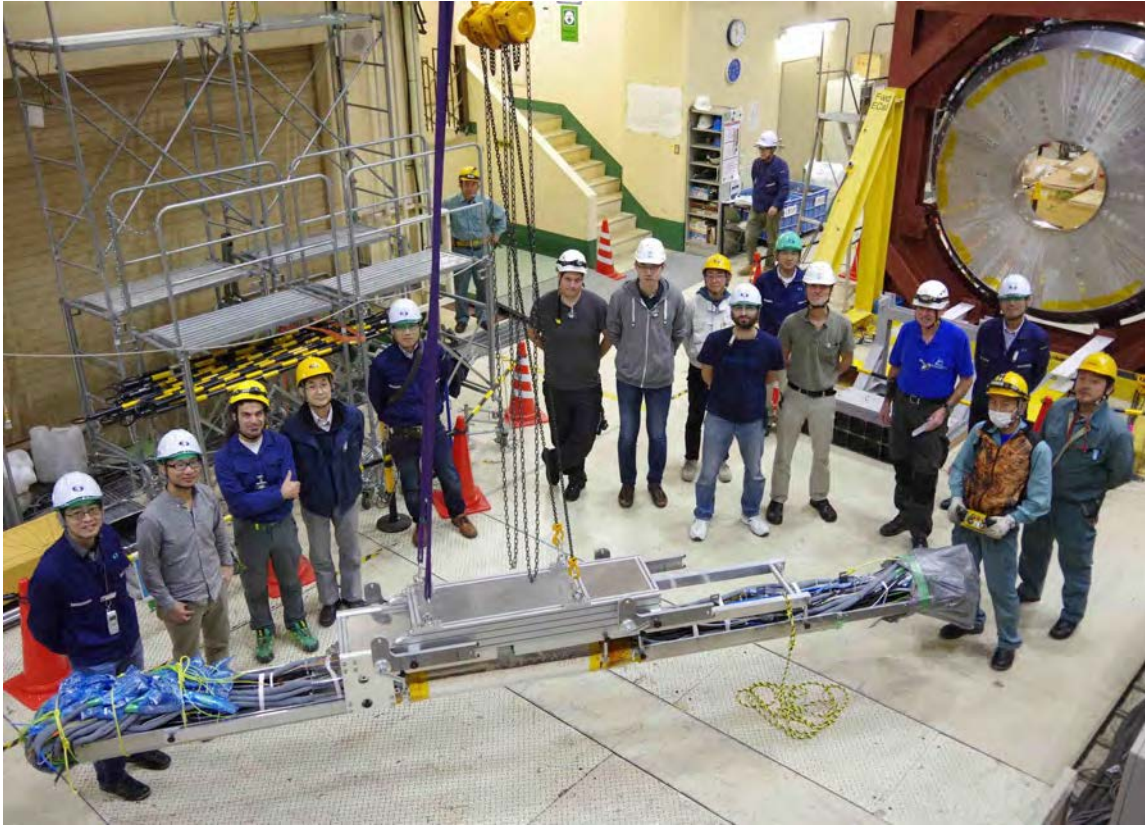
Figure 95. Photo taken during the VXD installation in the Belle II detector: lift-up of the VXD with a crane. The cables and pipes were fixed in the cables trays on both sides.
