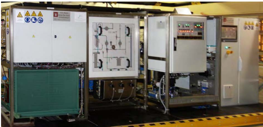
Figure 75. The IBBelle cooling plant. The four chassis from left to right are for the R404A refrigerator, the CO 2 pumps and tubing, the accumulator, and the control unit. In total, the cooling plant occupies a 6 \times 1.5 \times 2 \text{ m}^3 volume.
