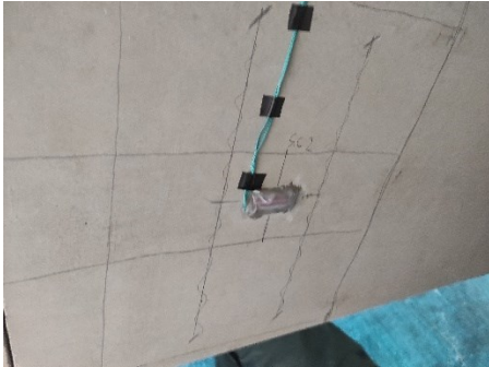
Figure 4-32: Identification of reinforcement and mark of cuts to be carried out at a distance of 12 cm.
