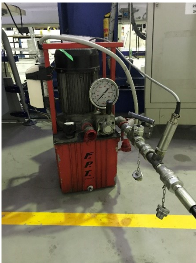
Figure 3-57: Oil pump of the ring hydraulic jack.
