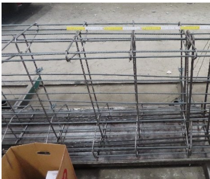
Figure 3-2: Stirrups \varnothing 8/300 mm shaped like the "I" section in the central area.
