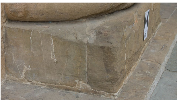
Figure 3. Detail of the calcite veins on the base of the Doric Order half column (May 2021).
