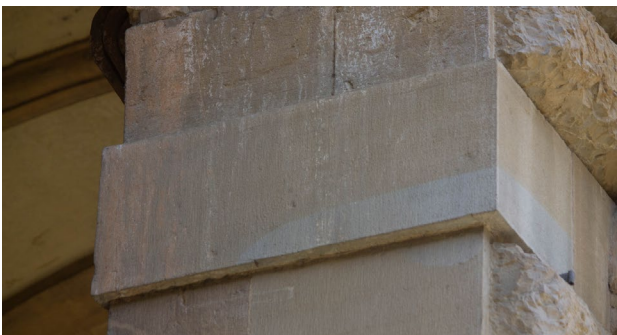
Figure 2. Detail of the impost ashlar of the Doric order arch showing the original colouring (May 2021).
