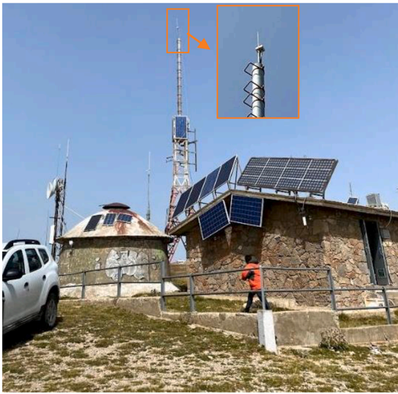
Fig. 9. Site for current detector installation: Eagle Nest Tower.
