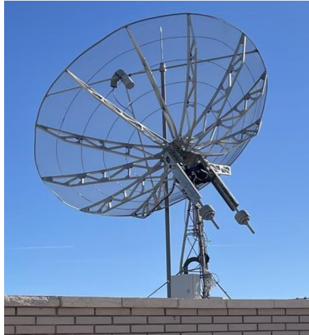
Figure 2.12: S-Band antenna installed at the OAdM. [20]
