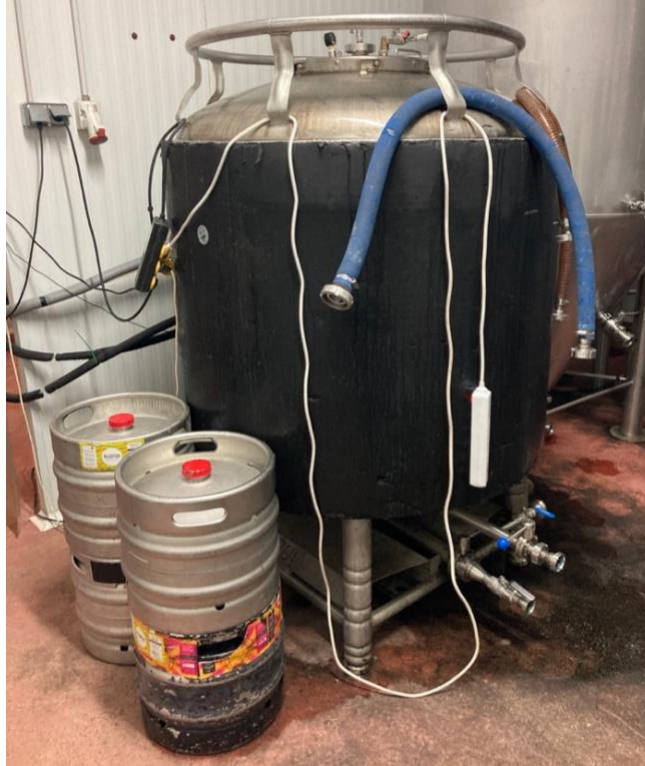
Figure 3.10. Secondary vessel where beer is carbonated
