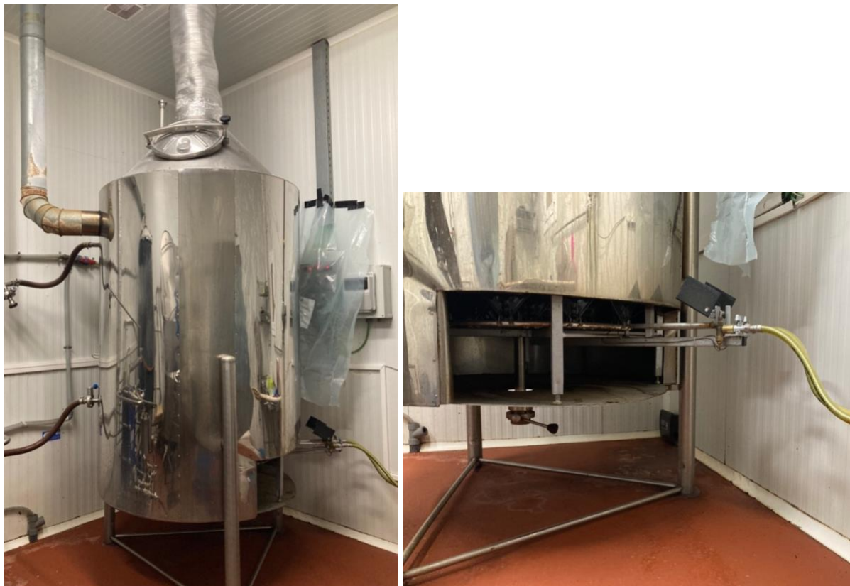
Figure 3.5 & 3.6. Kettle where the wort is boiled & entrance of the gas
